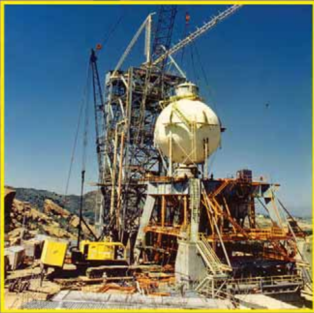
American 9299 Sky Horse Picking, Walking, and Setting 107-ton Spherical Fuel Tank at Rocketdyne Test Stand in California
