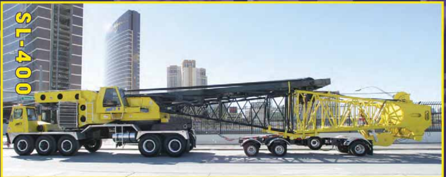
SL-400 Truck Crane Traveling Street-legal on Las Vegas Streets to Jobsite near Wynn Resort
